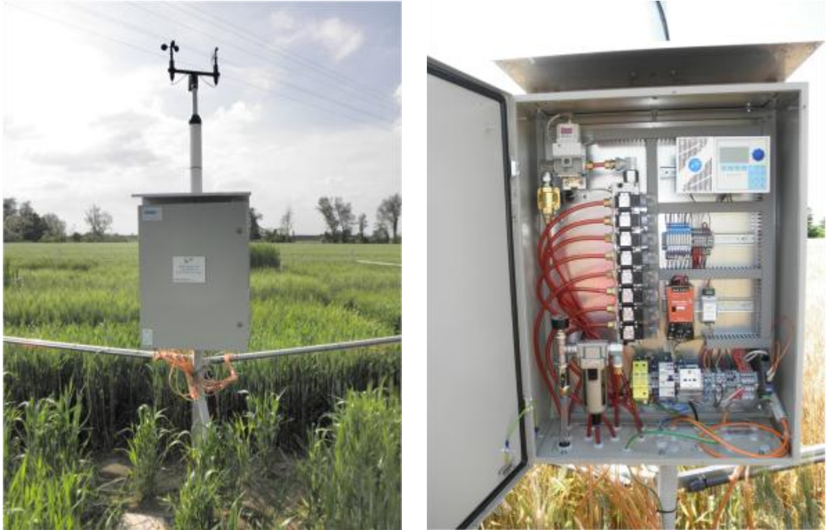
Fig. 7 Field installation showing the FACE controller mounted inside a water proof box which also contains the necessary hardware for the control of the directional [CO 2 ] release and the actuators.
